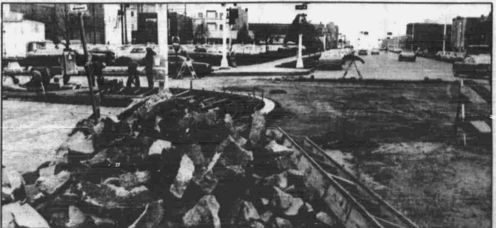
Downtown street project completion has been held up recently because old utility lines needed replacement. Photo by Bob Pearson
