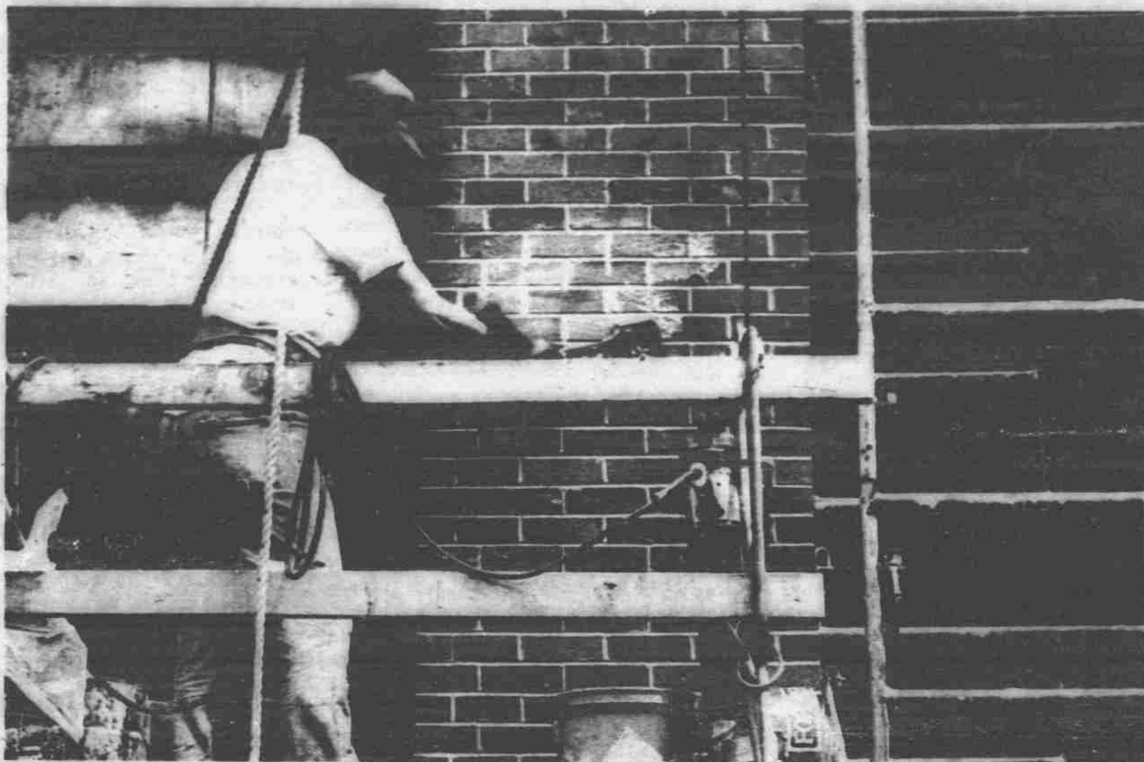
Joe Marostica, M.W. Anderson Co. employe, washes each brick as exterior work on UNL's Life Sciences Bldg. nears completion.
