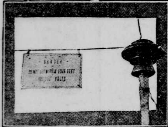
STYLE OF POLE, INSULATOR, DISCHARGE WIRES, AND WARNING SIGN ON ELECTRIC FARM
