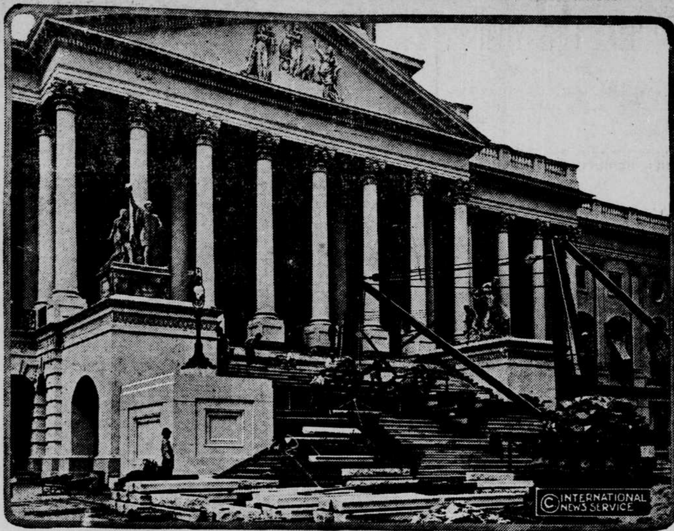
Workmen putting in new marble steps at the capitol at Washington to replace the old sandstone steps which time and the weather had rendered unsightly.
