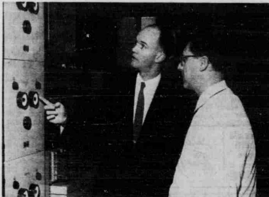
Roy Vaughn (left) discusses a central office power installation with Switchman R. F. Heider.
