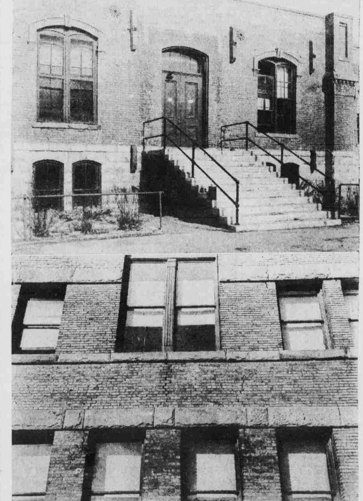
These photographs need no detailed editorial interpretation. The top picture, the entrance to University hall, effectively displays the many iron braces installed in 1925 to keep the building from caving in. The lower picture, the two floors of Nebraska hall, shows the cracking in the walls from a slipping foundation and decaying materials. On the roof of the same building are faults six inches deep where one wall has sunk in its foundation. Bars are also necessary to hold this classroom building together. Top floors of both buildings were torn off over ten years ago because of construction cavens.
