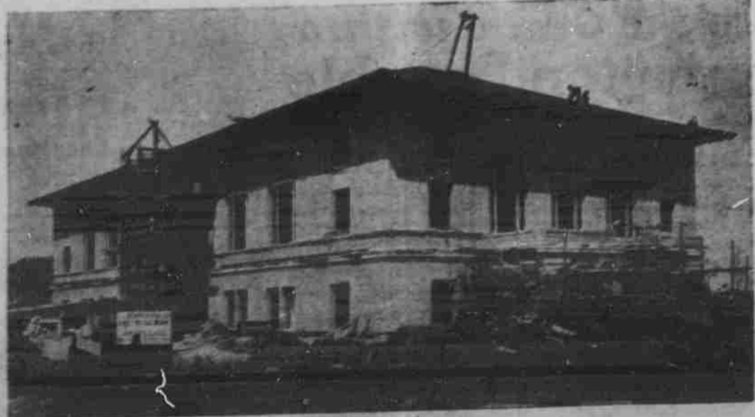
Due to the great expansion of the college of agriculture in the past few years, it has been necessary to erect a new activity house on that campus.
